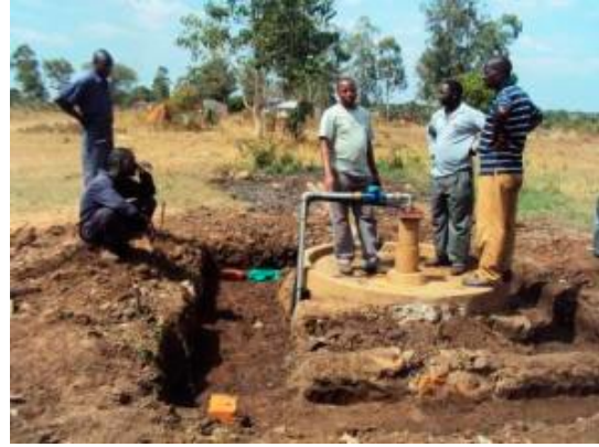
Picture 6. 14: An existing borehole installed with a solar pump in Oyam
