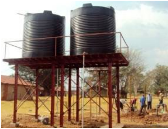
Picture 6. 15: Reservoir tanks for an institution in Oyam
